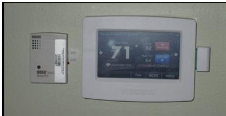
Figure 3. U10 Temperature Logger Installed Next to a Thermostat
